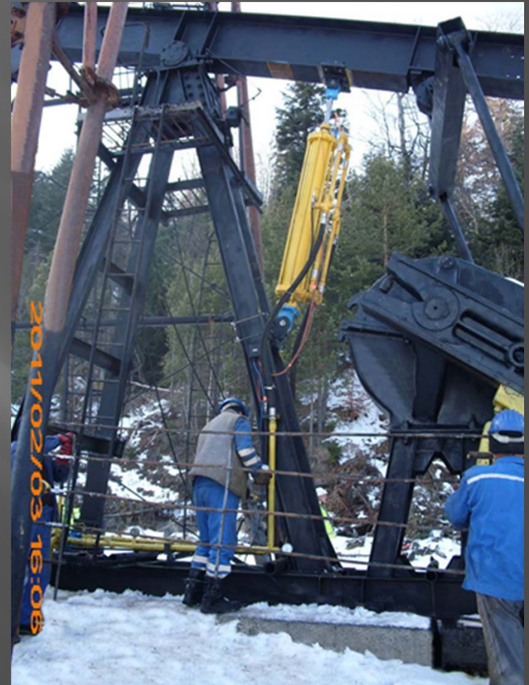
CGA 8x56 installation on a pump jack, Tașbuga formation
