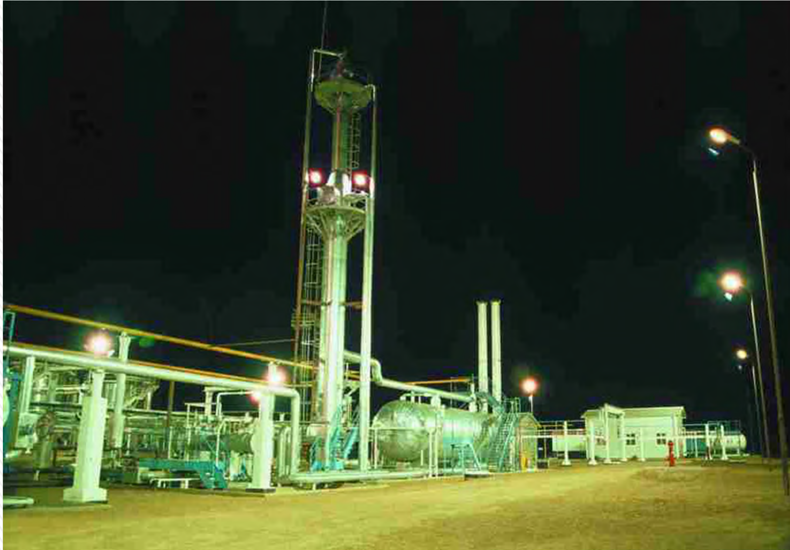
Condensate stabilizing column
