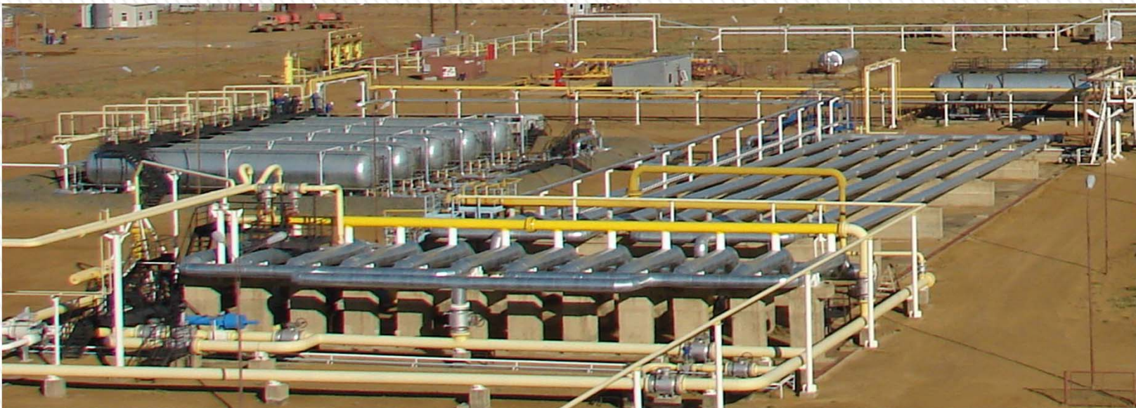
Propane storage tanks
