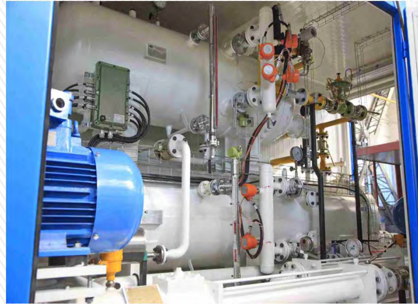
Three phase and bi-phase calibration separator
