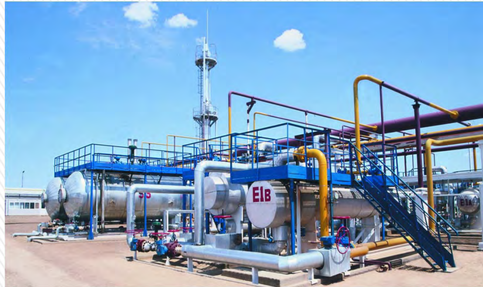
Three phase separators and heat exchangers
