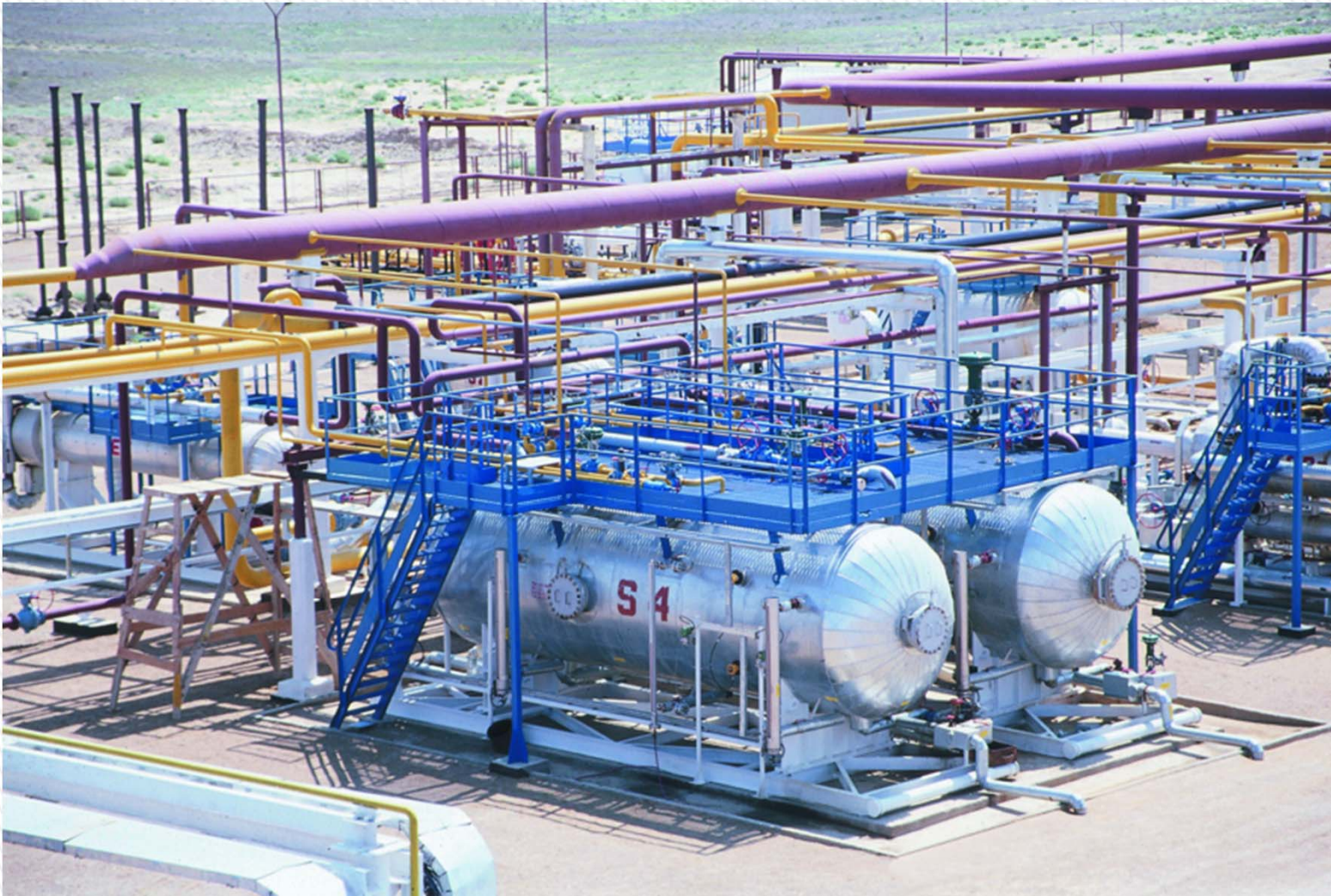
Three phase separators
